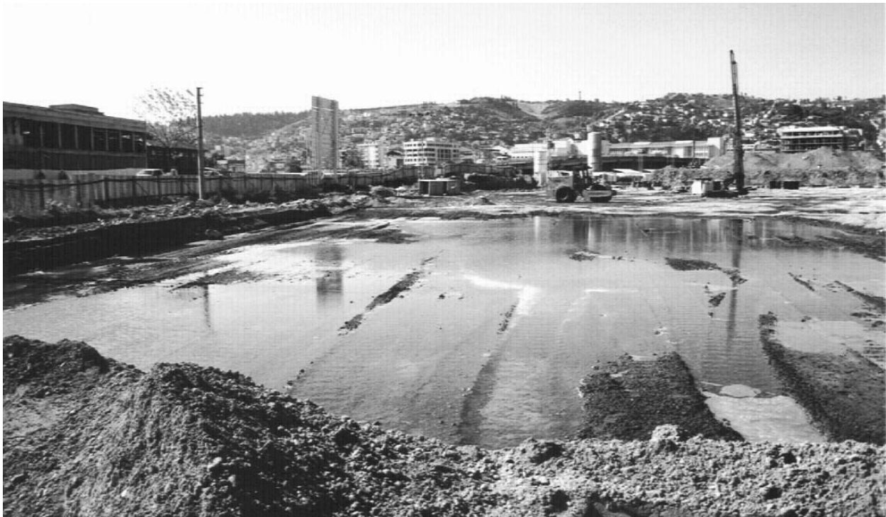
Figure 3. Ponding of water at portions of the parking structure area that were not yet treated with jet grout columns, Lot C under the preload fill is visible at the back – photograph taken the morning after the earthquake from the site border looking north
